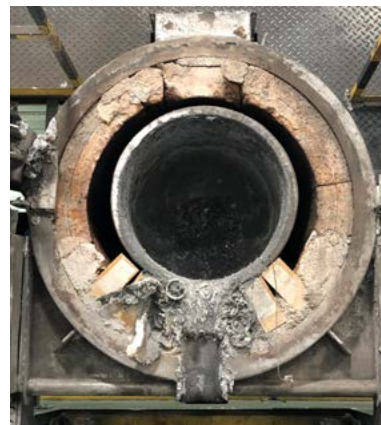
Figure 5: The DURATEK Supermelt after 1284 melt charges.
